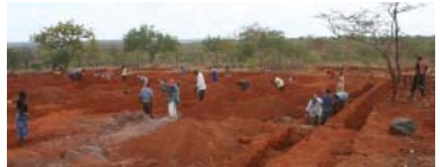
The Village at Kitui is taking shape as workers turn arid ground into a place of hope.
